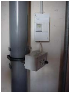
Fan and variable frequency controls
